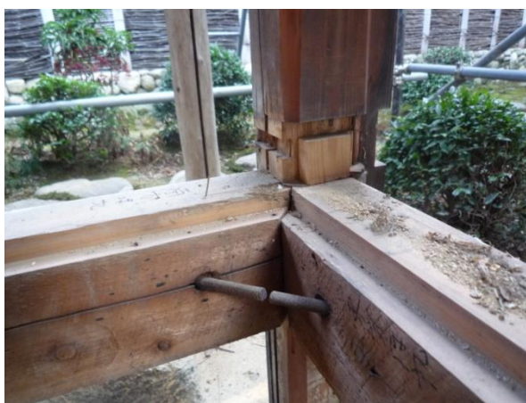
Fig.5) Dismantlement and reconstruction in a new site; connection of the pillar with the threshold sill.
