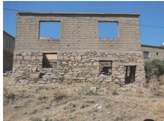
Fig 14. House with roofs collapsed in Çevre Settlement.
