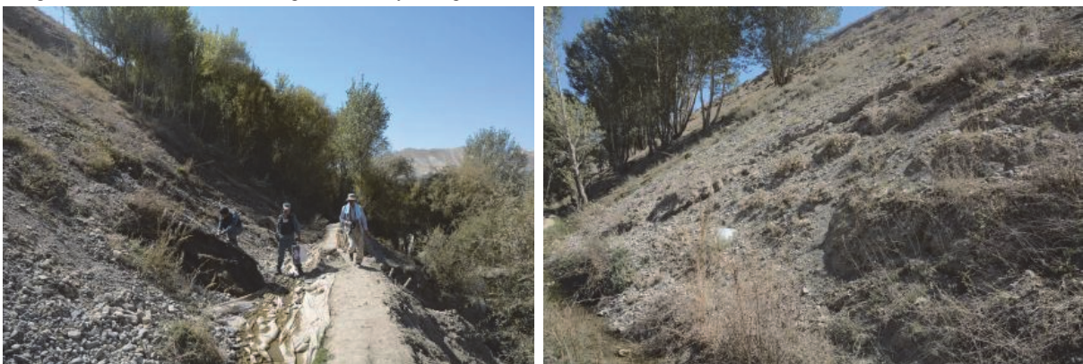
Waterway along the slope on the north side of the planed area (Left: waterway, Right: slope)
