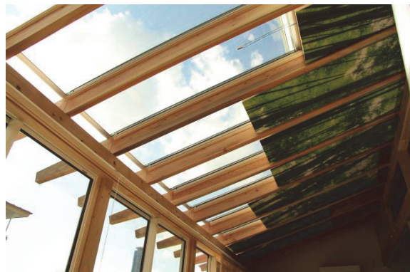
Figure 9 Highly insulated shades under skylights that can be moved up and down manually or via electric power.
