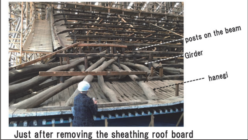
Figure 47: The long sloping logs called hanegi holding up the eave at the restoration site of Honryu-ji Temple, Kyoto.
