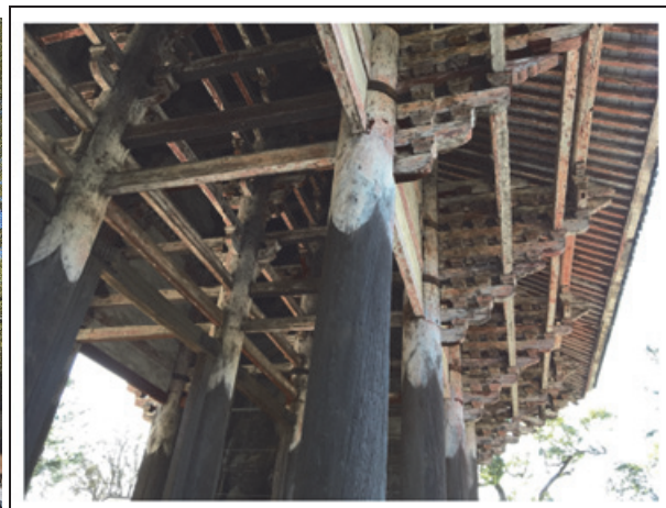
Figure 14: All Frames are exposed.
