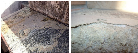
Figure 4 Defects of the stone materials (left: Nikka stone, right: Tatsuyama stone)
