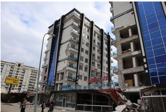
Photo 1-4 Onikişubat, K.Maraş. Peeling of exterior walls of apartment buildings.
