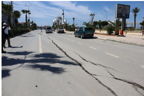
Photo 1-61 İskenderun, Hatay. Fissures in the ground
