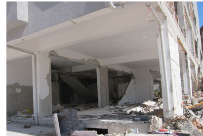
Photo 3-3 Column Flattened in the Storefront Direction
