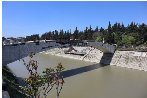
Photo 1-27 Antakya, Hatay. Peeling of bridge finishing materials.
