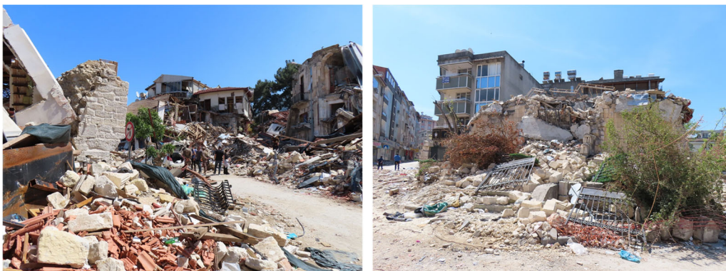
Photo 2-10 Seismic damage in Antakya old urban area
