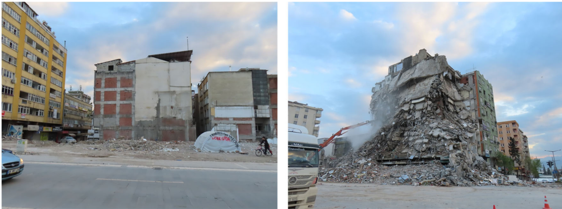
Photo 2-8 Seismic damage in Kahramanmaras (Location ⑥)
