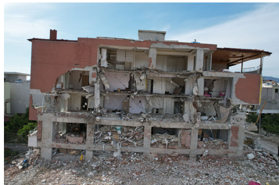
Photo 1-51 Samandağ, Hatay. This was originally a six-story apartment building. The first and second floors were crumbling.
