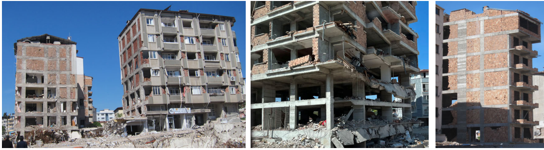
Photo 3-4 The Damaged RC Buildings (Left) and Under-Construction RC Buildings (Center/Right)
