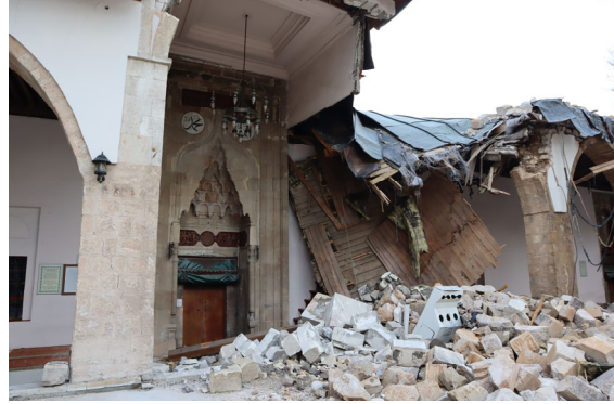
Photo 5-2 The entrance area was damaged.
