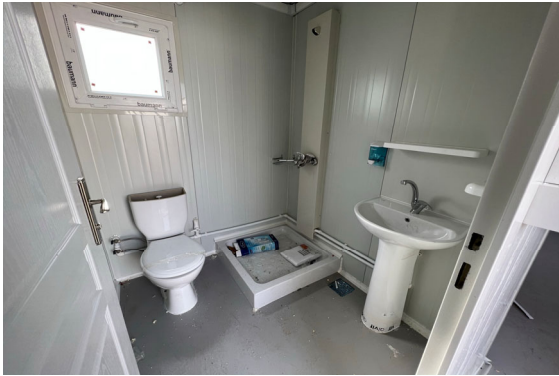
Photo 4-17 Inside the container. Toilet, shower and hand wash.
