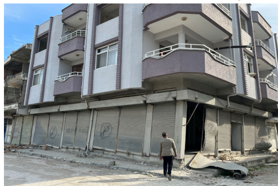
Photo 1-53 Samandağ, Hatay. A building whose layers were collapsing.
