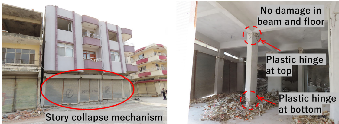
Photo 2-11 Seismic damage in Samandag
