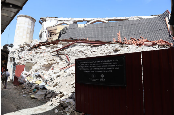
Photo 5-23 Antakya, Hatay. Mahremiyeh Camii. The minaret collapsed.
