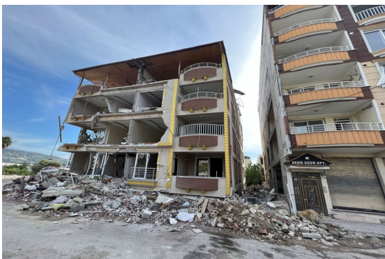
Photo 1-52 Samandağ, Hatay. Photo from another angle. Originally bordered by the neighboring building.
