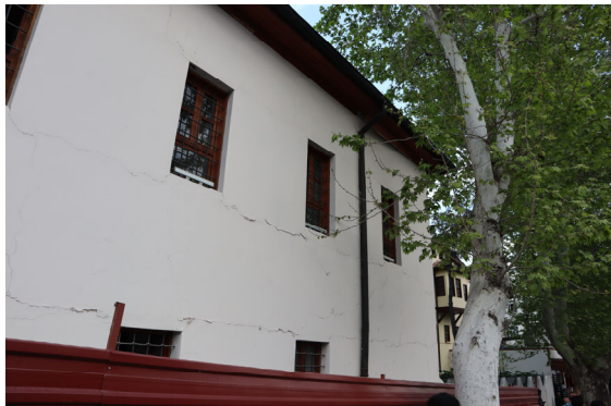
Photo 5-16 Cracks in exterior wall.
