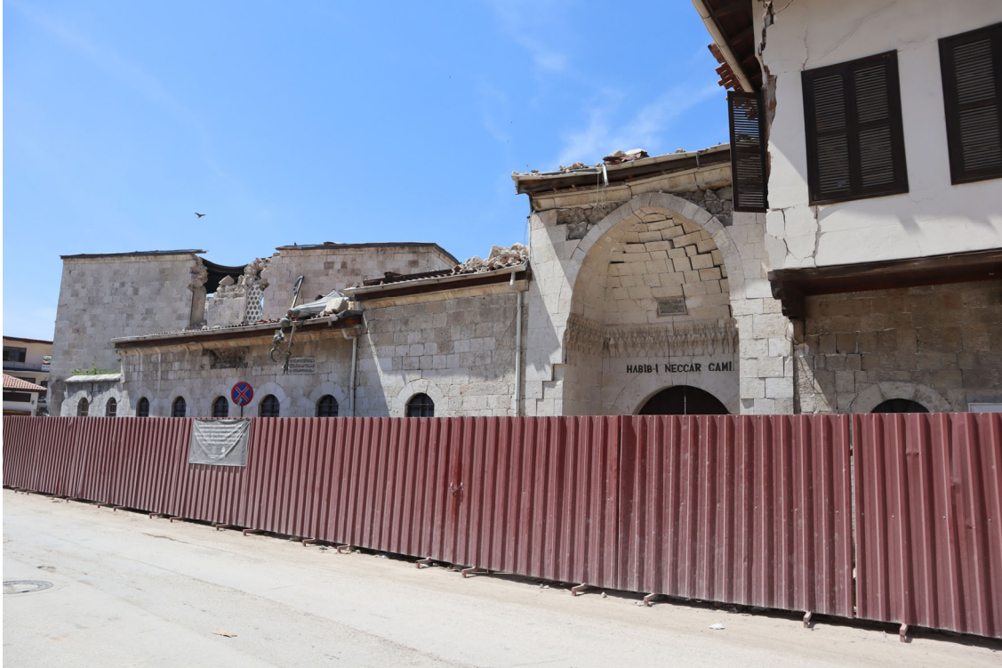
Photo 5-22 Antakya, Hatay. Habib-i Neccar Camii The minaret and dome collapsed.
