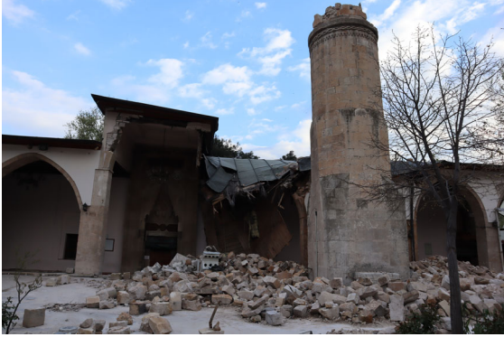
Photo 5-1 The minaret collapsed and stones were lying on the ground. The entrance area was damaged.
