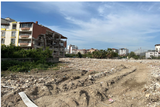
Photo 1-50 Samandağ, Hatay. Site where an extension building collapsed.
