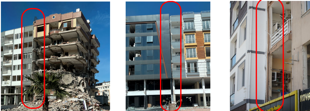
Photo 3-1 Adjacent buildings in close contact
