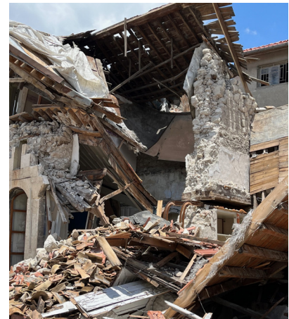
Target house: The collapsed east gable wall of the second-floor extension
