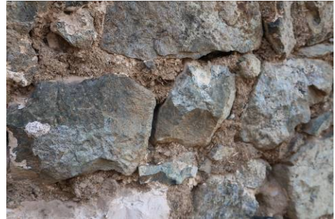
Poor earth mortar
